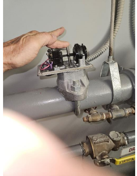
Manually Operating Switch
