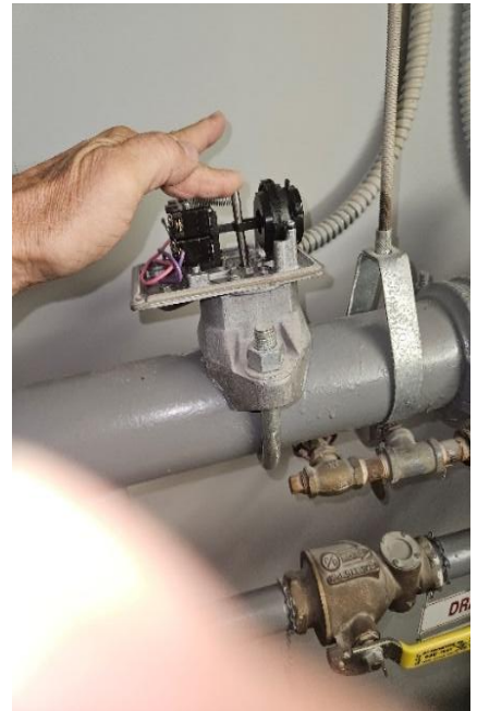
Manually Operating Switch
